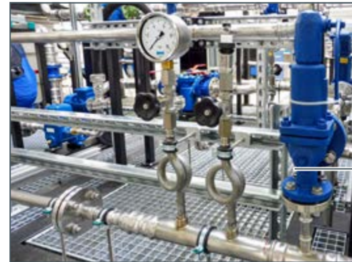
The operating parameters are monitored with the aid of measuring instruments
