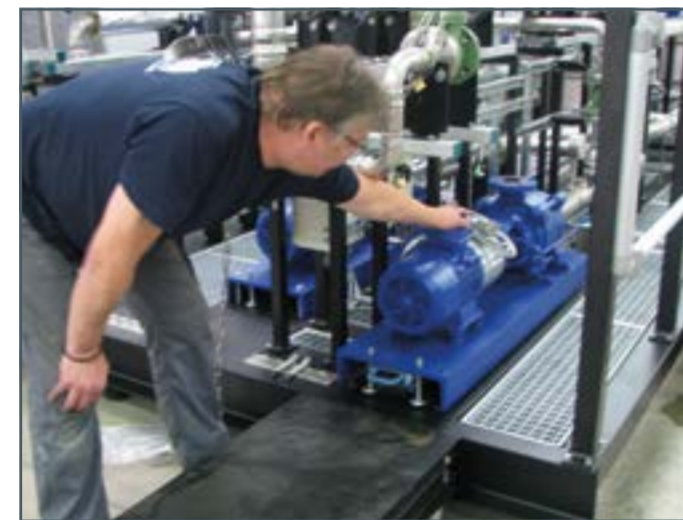
Pumps can be removed and tested
